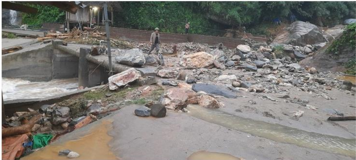
Figure 2.3 Severe flash flood in Lien Minh commune, Sapa town, Lao Cai province on the evening 12 th September caused 8 peoples dead and missing
